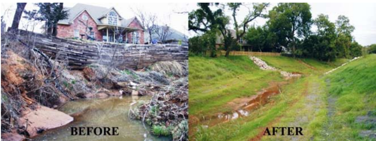
Figure CS16–10 Eroding channel prior to construction, and after project implementation; house and property lines imposed restrictions on the design
