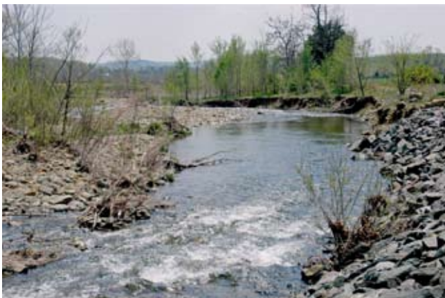
Figure CS5-15 Raw bank downstream of riprap
