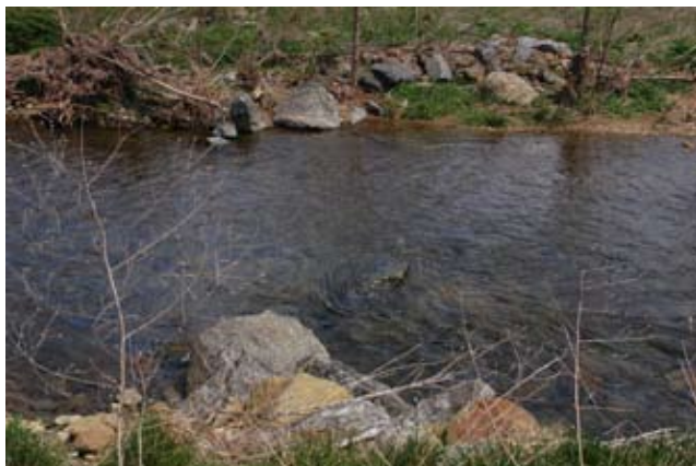
Figure CS5-12 Weir #7, April 2004, after Hurricane Isabel
