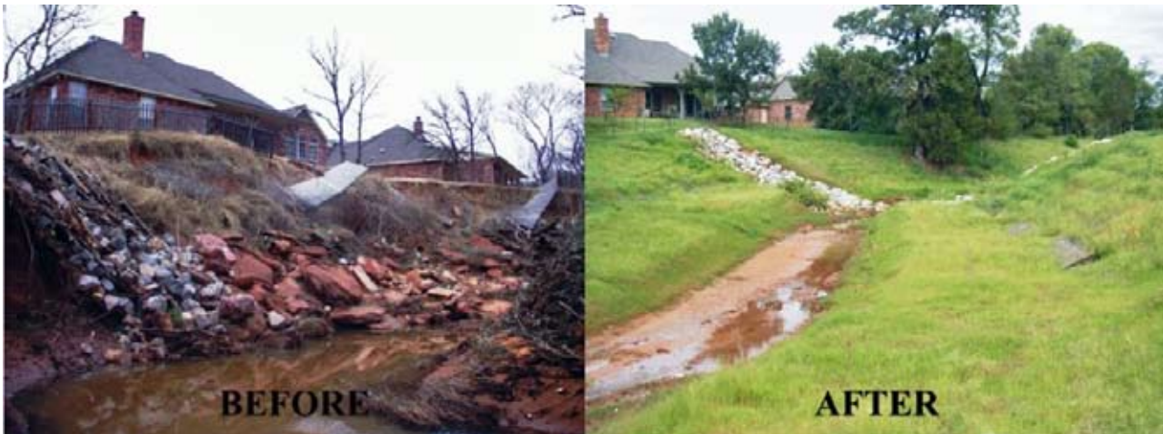
Figure CS16–9 Eroding channel prior to construction, and after project implementation; house and property lines imposed restrictions on the design
