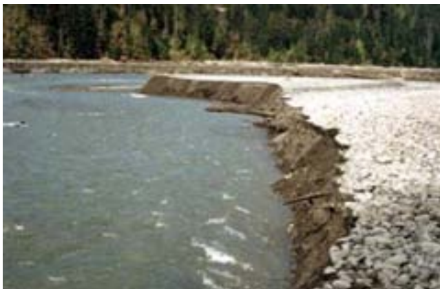
Figure 7-9 Degradation through armor layer
