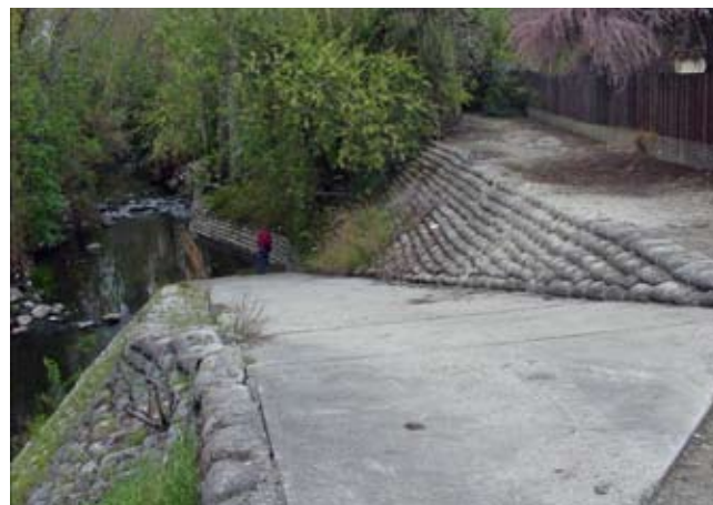
Figure CS15-1 Damaged access ramp and wall
